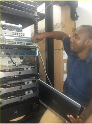
IT staff in one of the Unit server rooms
