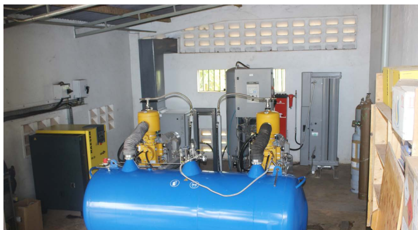
Nitrogen plant - Entebbe UVRI Campus
